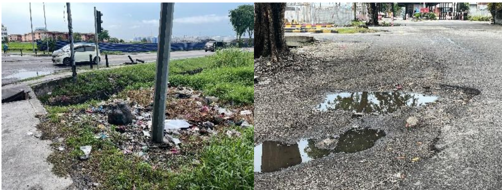
Figure 6. Examples of deteriorating public infrastructure and environmental maintenance issues observed in Southport. Source: Field observation by authors (2026).
